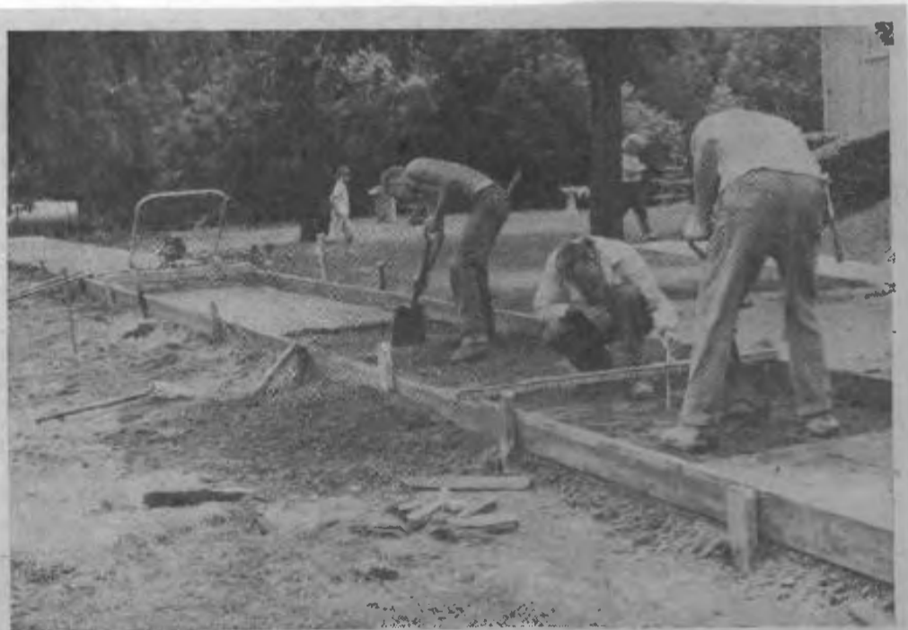
CONSTRUCTION BEGAN last week on the $54,000 Wheeling sidewalk program. The 3.2 miles of walks are to go along Wolf, Dundee and Elmhurst Roads. Work began on the Wolf Road portion. (W)
