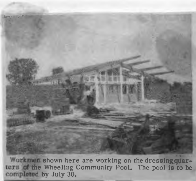
Here is a shot of the soon-to-be-completed Wheeling Community Pool on Wolf Road near Chamber of Commerce Park.
